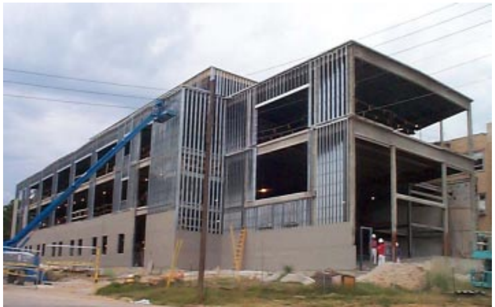
Cold-formed steel framing being used in the renovation of the Bulter-Carlton Civil Engineering Hall at the University of Missouri-Rolla. The Center offices and technical library will be housed in the front section of the third floor which can be seen at the right in the photograph.
